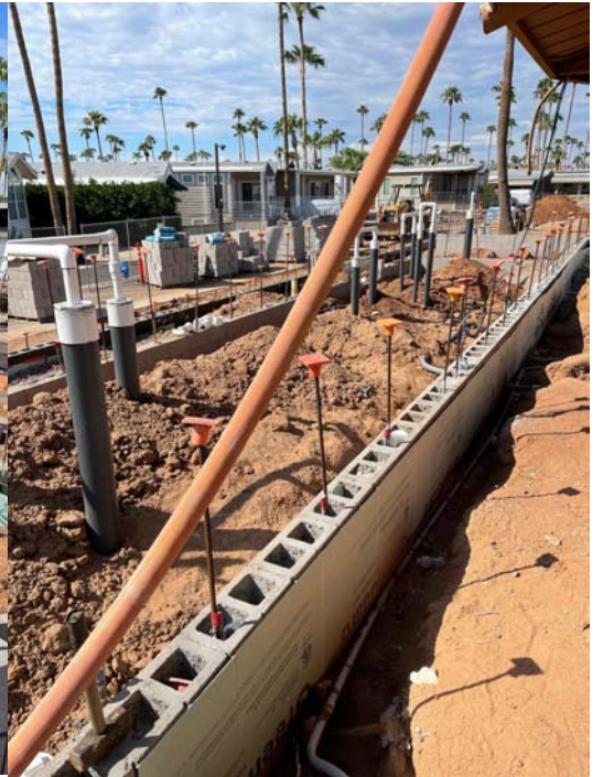
Same pump house west pool.
