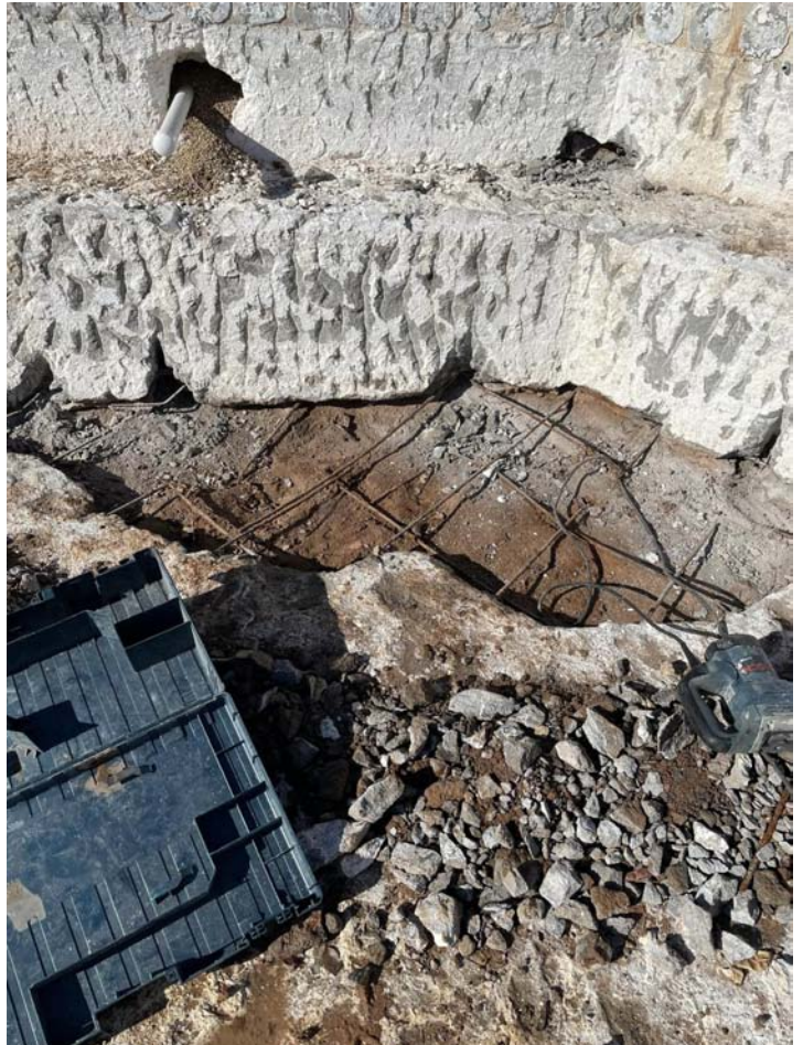
More examples of rusted rebar
