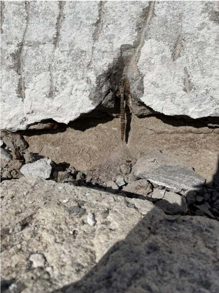
Best example.. very rusted rebar like a rotten tooth .. all of this has to be removed until we could find good rebar
